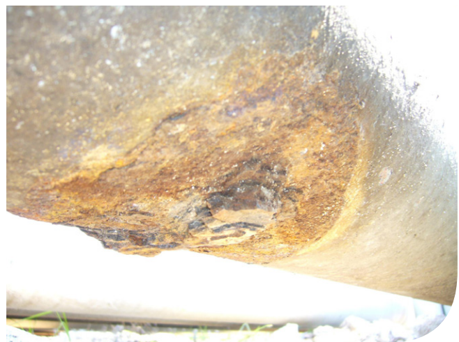
Example of corrosion in a pipe
