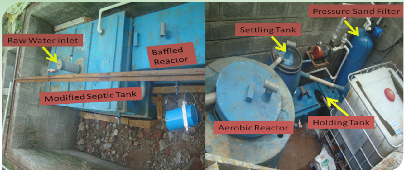
Photographical view of on-site waste-water treatment.
